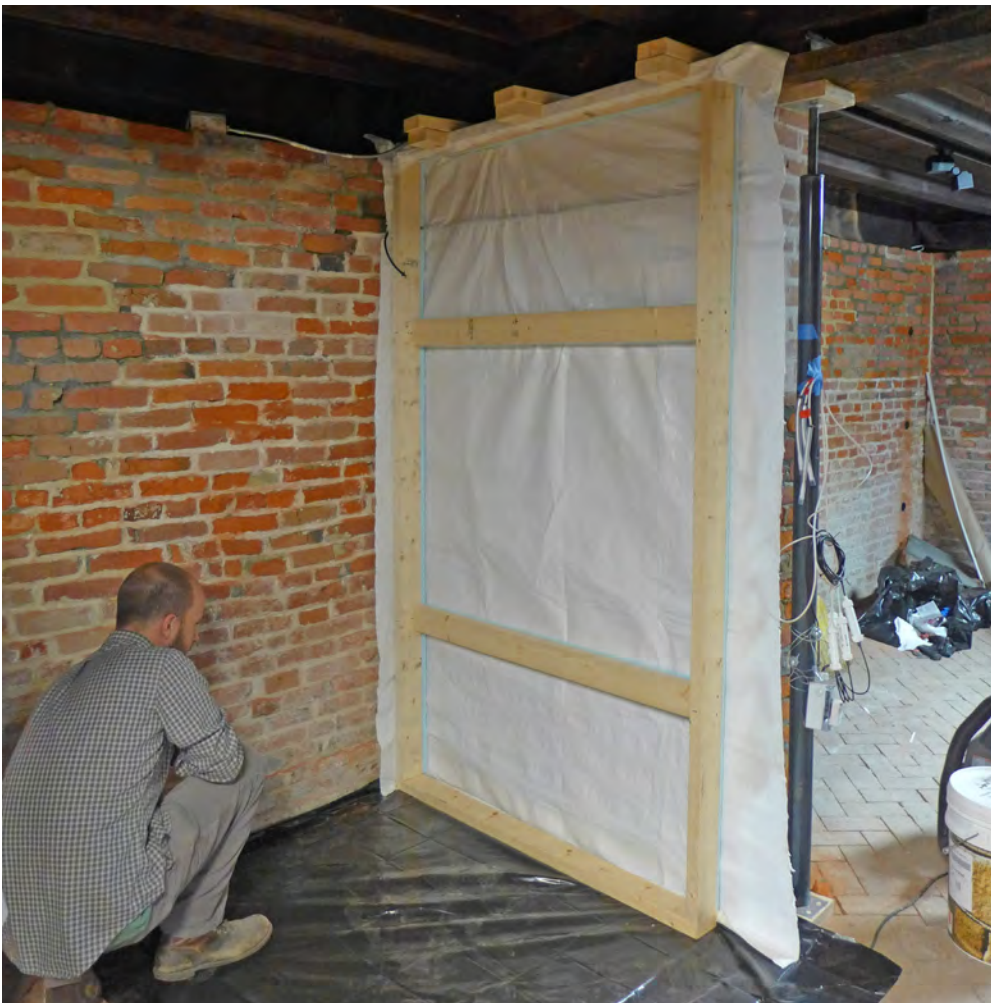
Image 12: Wet curing blanket and frame installed at wetting side of the test wall.
