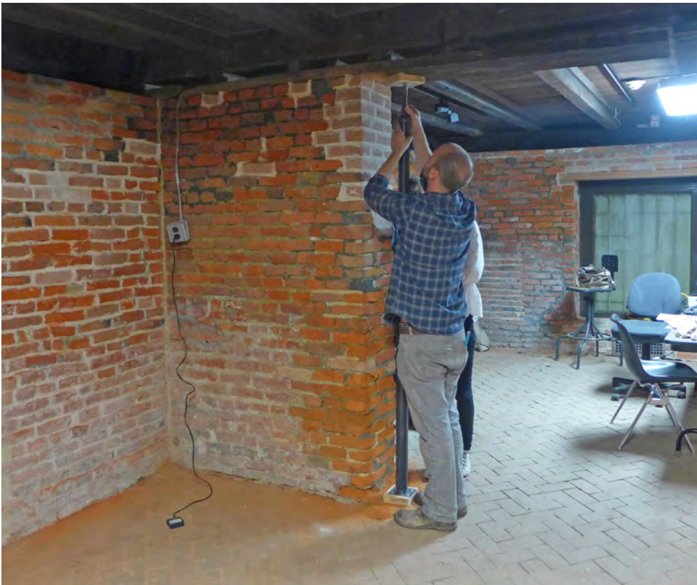
Image 6: The wood member on top of the wall was supported by a steel column before the start of the treatment.
